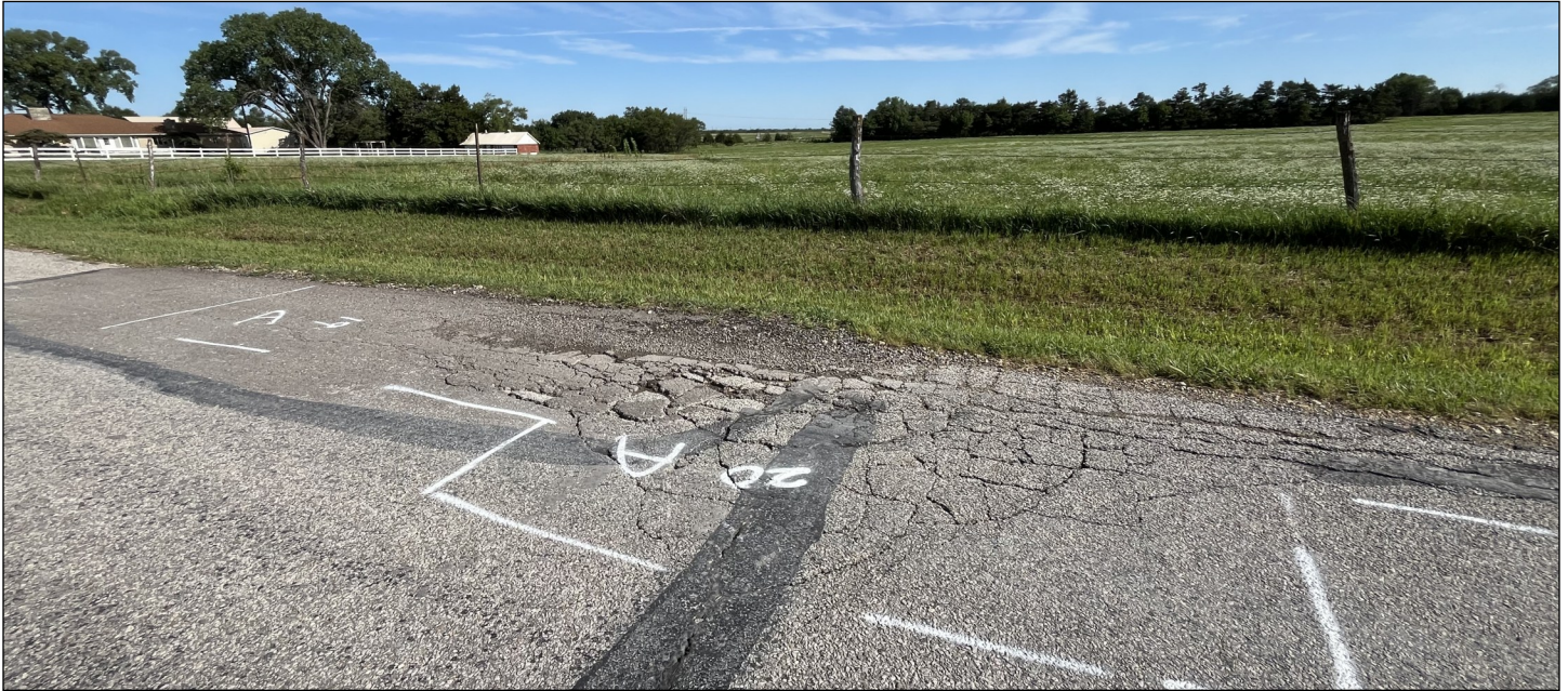
“Alligator” pattern cracking is marked for repair on Clay Hill Road. The marked sections of Clay Hill and 6th Street indicate places where failing sections of road base will be repaired to create a stable base before roads are resurfaced. Work began in late June and will continue into July.
